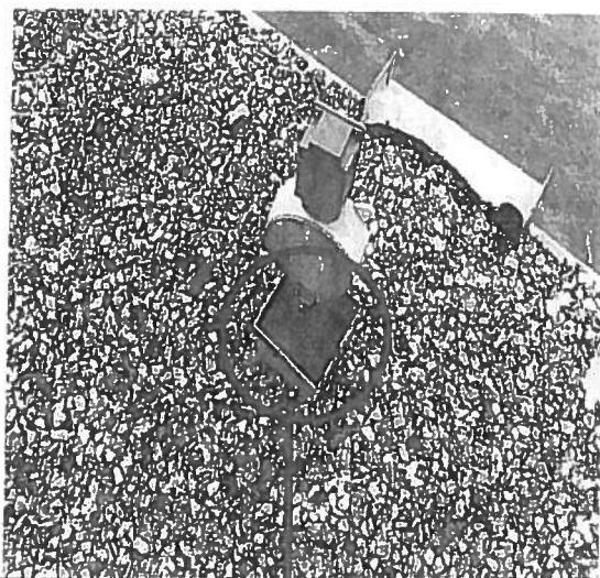
Inspect and redo pitch pockets with curbs around HVAC units on all roofs.
