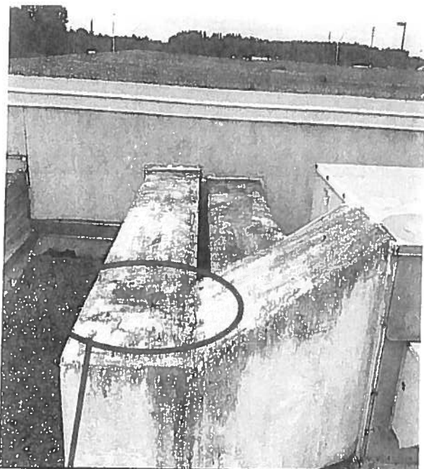
Reseal rooftop air conditioning duct with fab tape and mastic. Rainwater is penetrating the existing ductwork causing leaks inside the building.
